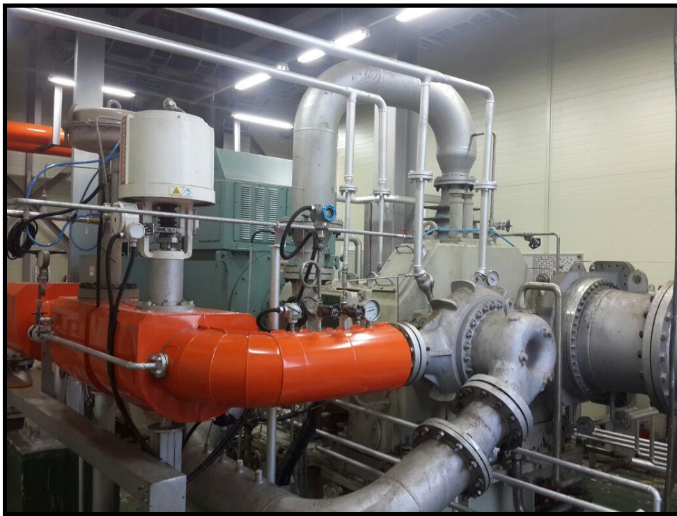
3 MW Capacity ECT™ at Water Incineration plant in South Korea
